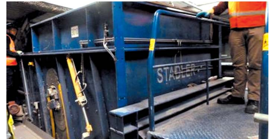
Case 3. This ballistic separator, which separates organic and inorganic waste, had not been isolated from the power supply when cleaner climbed into the top level. The machine was switched on from the control room and he was fatally injured.
