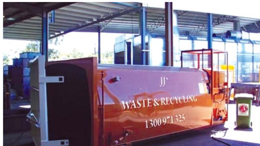
Case 2. This machine is used to compress recyclable and waste materials and has a defeated interlock system enabling a worker to enter the machine while still in operation. The worker had entered the baling chamber to clear a blockage of waste materials that had caused the machine to stop. The machine automatically activated, and the worker suffered fatal injuries.
