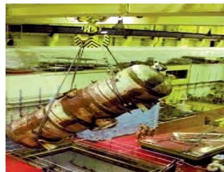
Case 1. An unsupported metal section weighing approximately 1.3 ton fell on a worker and fatally crushed him
