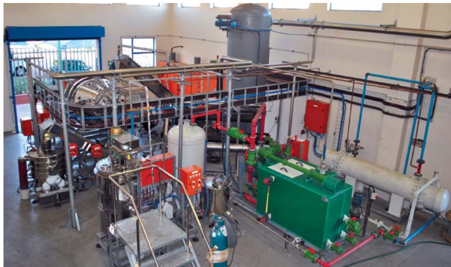
Carbon Impregnation Plant
